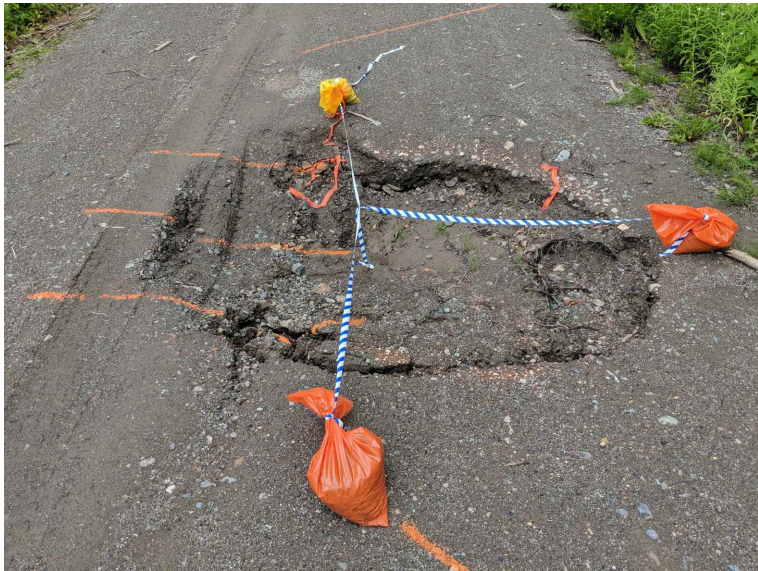
Sinkhole in Road
